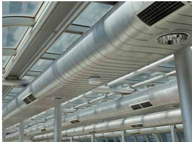
Intelligent demand control ventilation uses high quality sensors to accurately measure air quality to inform building ventilation controls and optimise ventilation effectiveness
