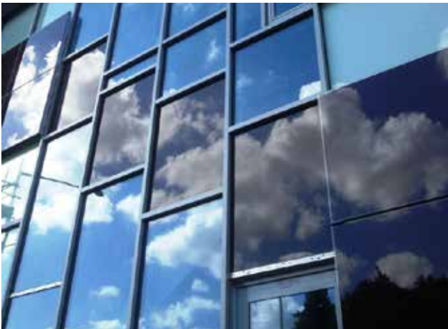
Solar PV glazing system at Future Business Centre building, Cambridge. The U-value of the integrated panels is similar to that of a high performing façade
